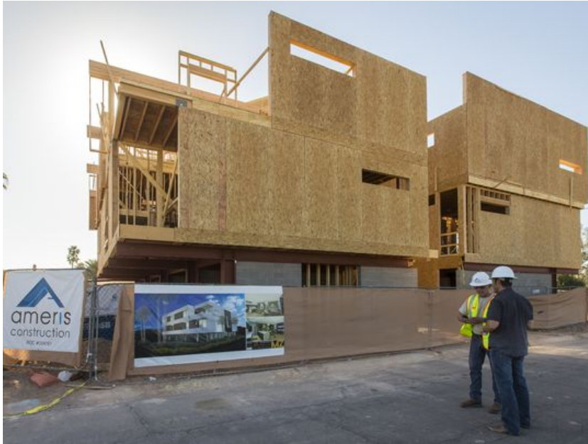
Work is well underway on the new eight-unit MZ condominiums northeast of Camelback and Scottsdale roads on Thursday, April 17, 2014. (Photo: Charlie Leight/The Republic)
